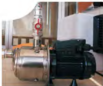
Electric pump connected hydraulically
